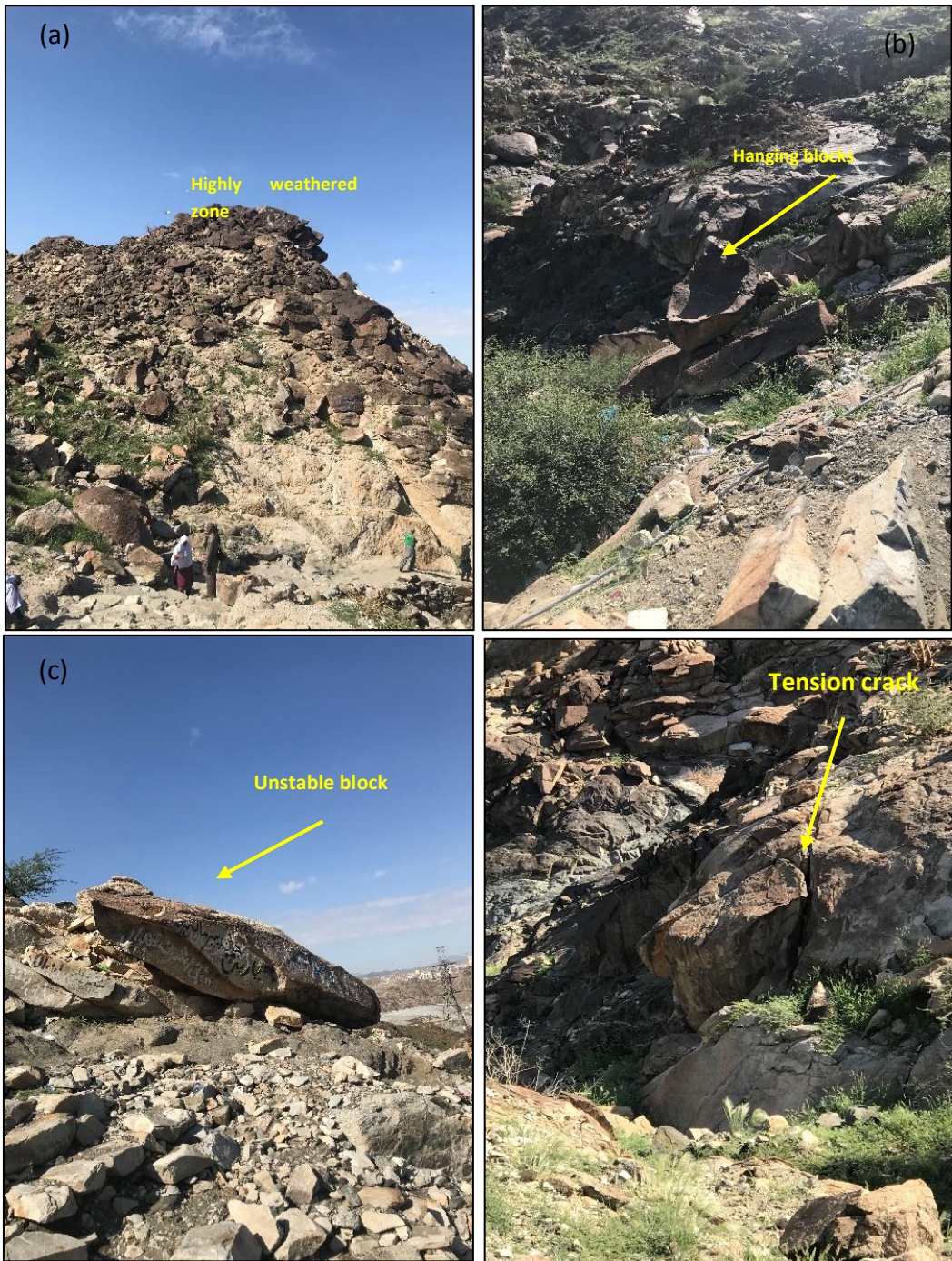
Fig.(8): Field photographs show (a) highly weathered granodiorite (b) unstable blocks and tension cracks structure at the road side (c) steep fracture planes at the road side, (d) small hanging blocks.
